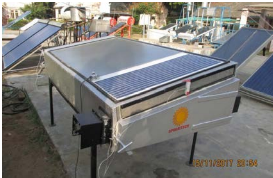
Fig. 5: Single module PV integrated low tunnel dryer
