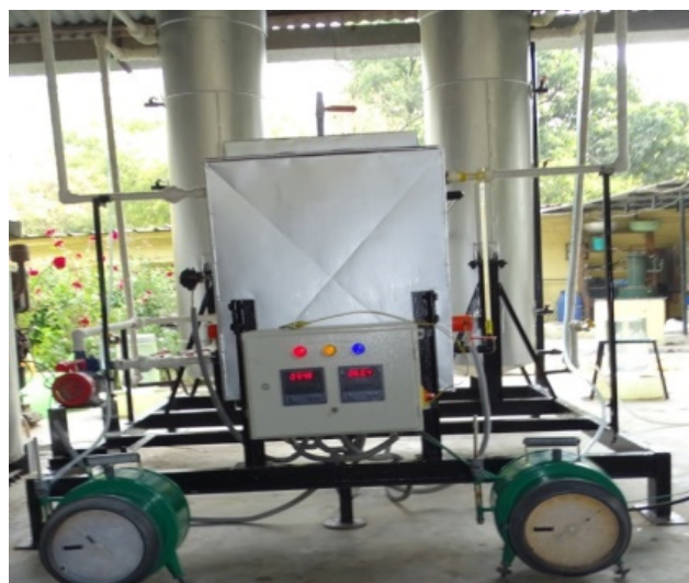
Fig. 4: Jacketed thermophilic anaerobic hybrid reactor
