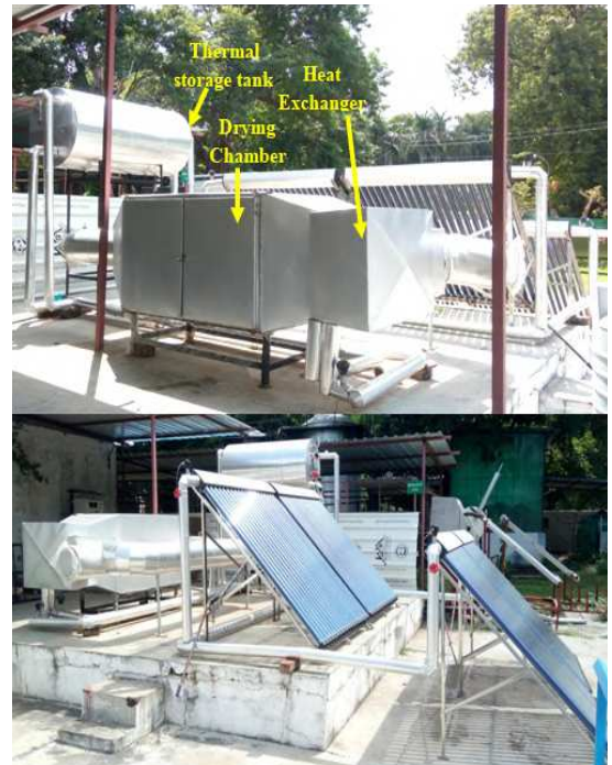
Fig.10 Front image and side image of installed solar ETC heat pipe and thermal energy storage based indirect dryer
