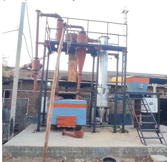
Fig.16: Fluidized bed gasification system installed at Swastik poha
