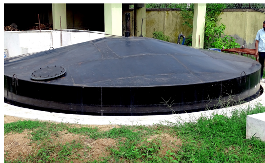
Fig. 40 Biogas plant at Vatsalya International School, Borsad
