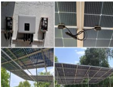
TPI for Solar Rooftop System
