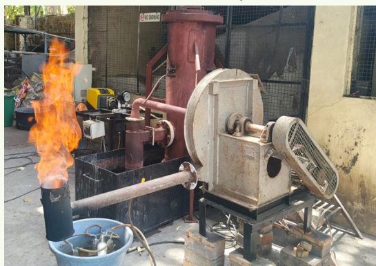
Figure 4.3: Downdraft oxy-steam gasification system under stable operation
