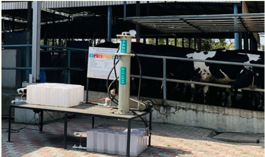
Figure 3.7: Bio-char-based bulk milk chiller effluent treatment system (100 LPH) site
