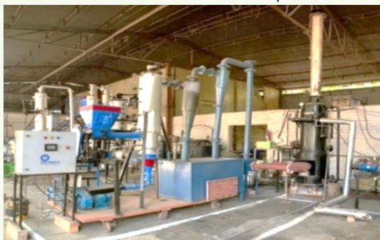
Figure 3.3: FBG unit with PLC-based automation for steam generation
