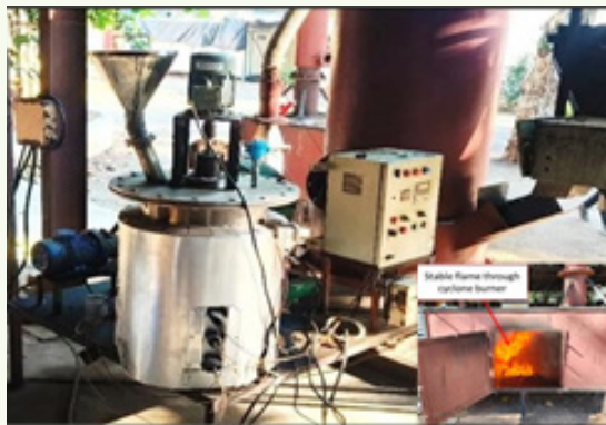
Figure 18: Bio-oil combustion unit and burner with stable flame
