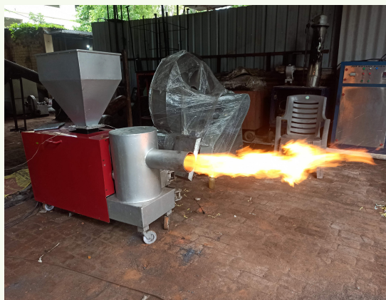
Figure 20: Pellet burner during operation
