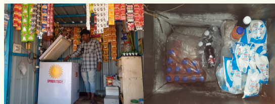
Figure 2: Refrigerator installed at user site for storing milk and cold beverages
