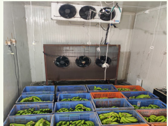
Figure 4: Load test of cold room with banana
